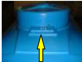
OUTER MANLID PADLOCK FACILITY
